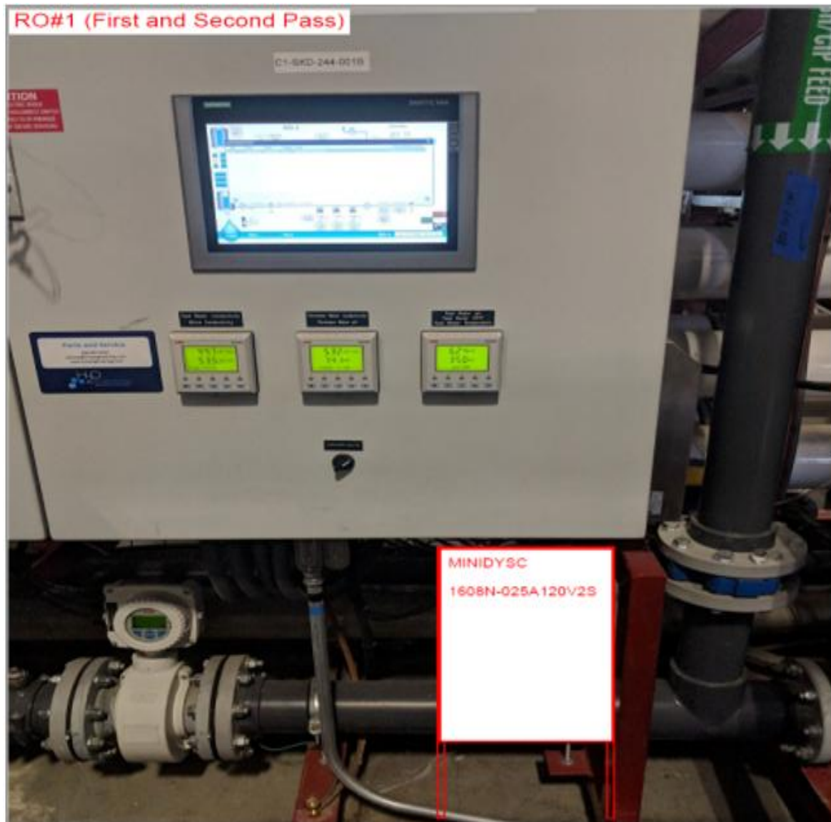
FIGURE 25: Site location of MiniDySC installation for RO skid.
