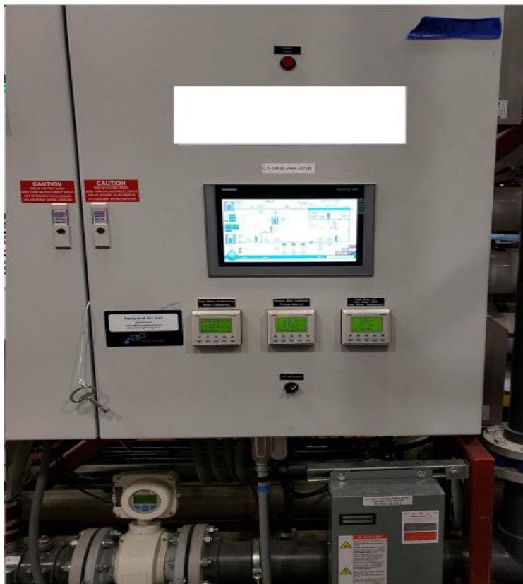
FIGURE 30: MiniDySC installation on RO skid.
